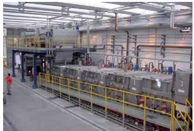
ESSETEX: drums washing unit
