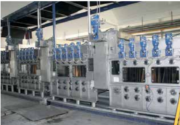
ACTIVA: cylinders washing unit
